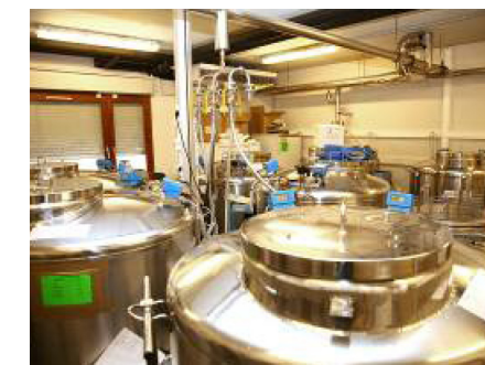
Fig. 3.9.6 Liquid nitrogen room
