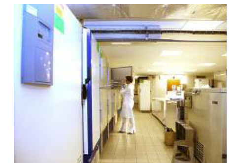
Fig. 3.9.7 Deep freezers room
