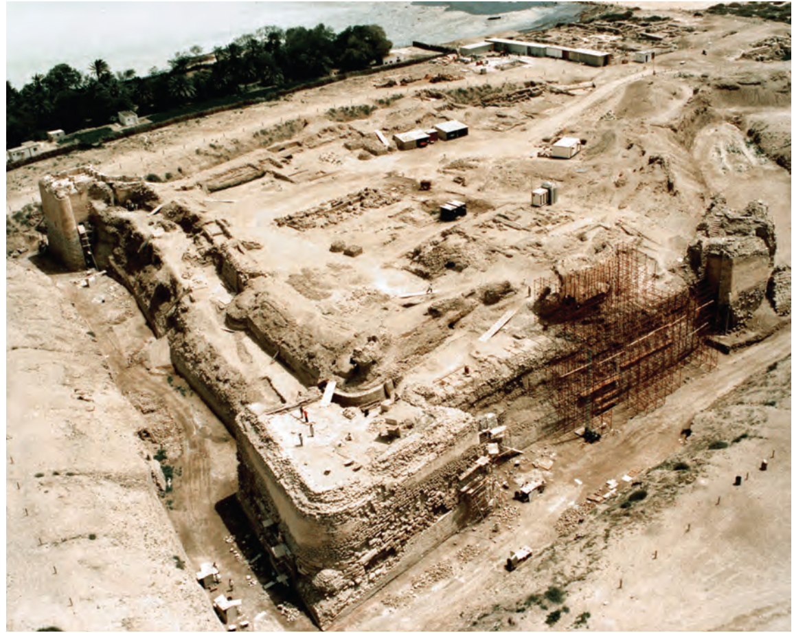
The Hormuzi-Portuguese Fortress ("Main Fort") under restoration by the Bahraini architects of the Ministry of Information (1988)
