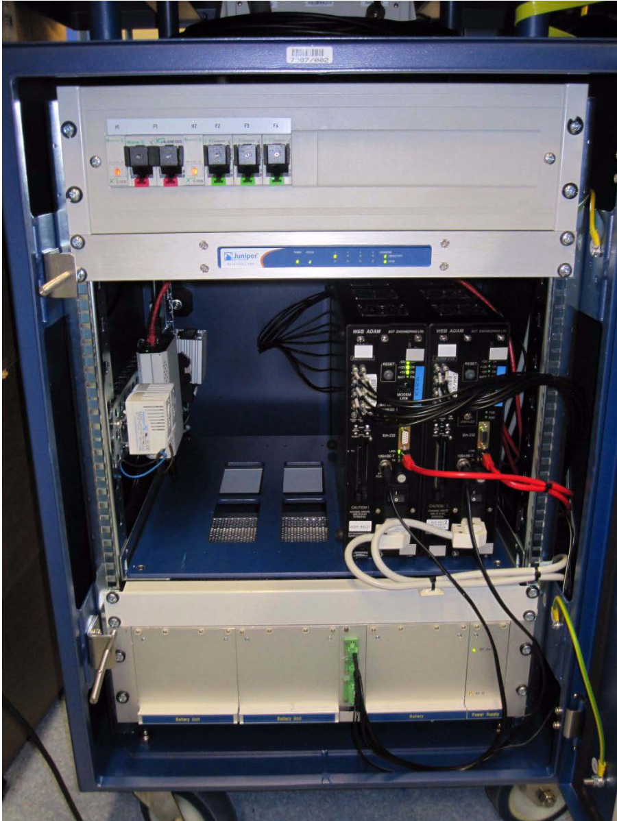
FIG. 22. Silo entry gamma monitor (SEGM) cabinet.
