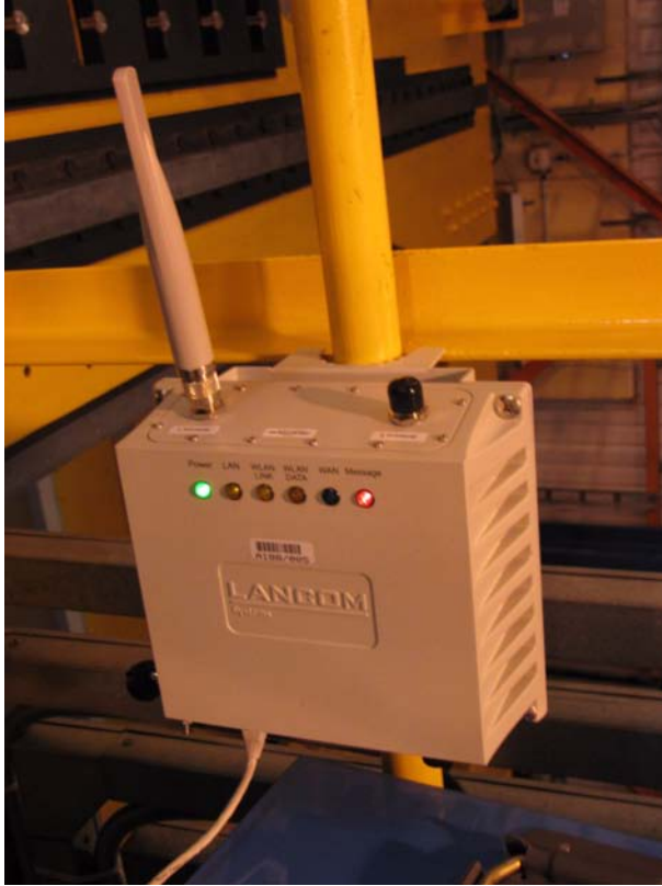
FIG. 44. Wireless communications equipment.
