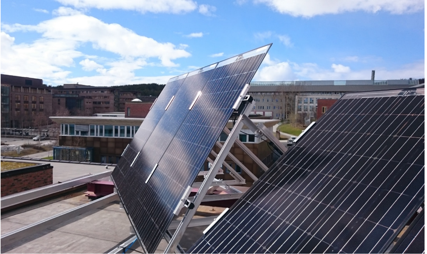
The solar panel system consists of 34 panels, each 1½ metres across; together, they cover about 55 m 2 of the roof. Nineteen of them provide electricity to grid and 15 will be set up to charge batteries. Photo: Clara Good
