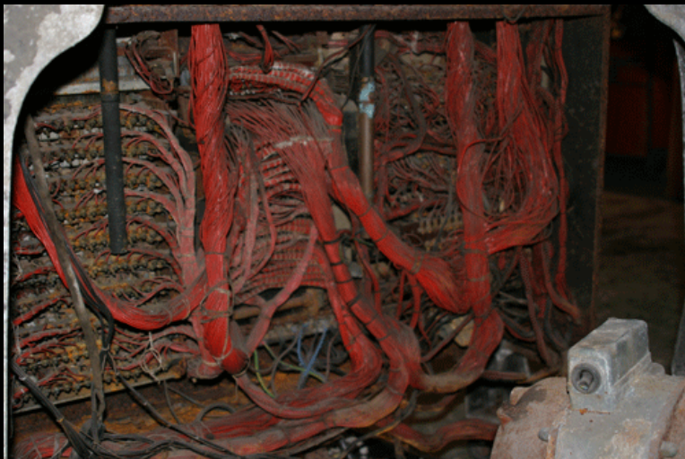
This is the back of the machine, showing all the control relays.
