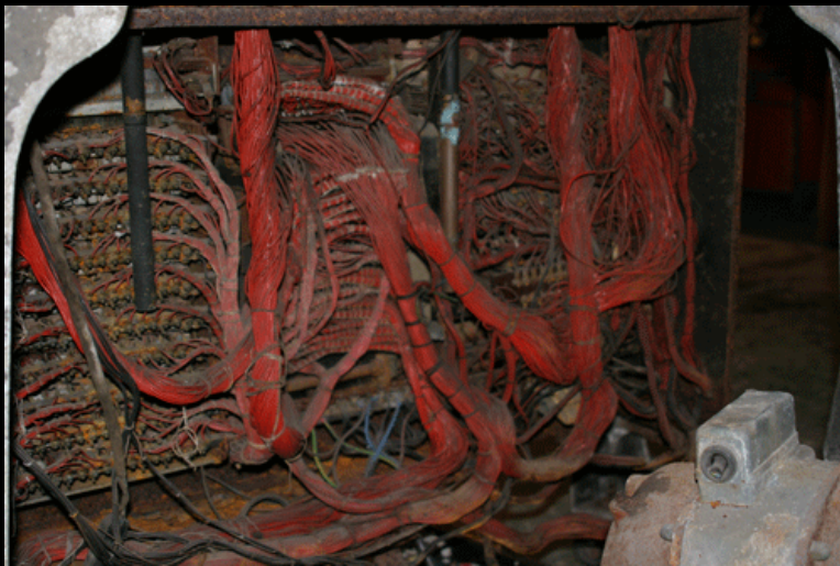
This is the back of the machine, showing all the control realys.
