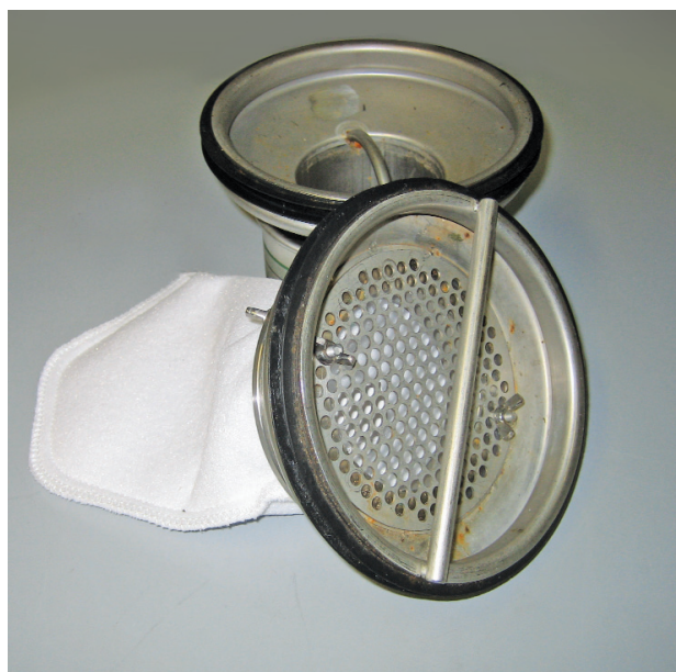
FIGURE 11. Filter Sock on Floor Drain*
