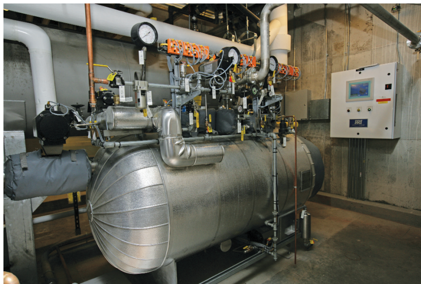
FIGURE 6. Liquid Effluent Sterilizer*
