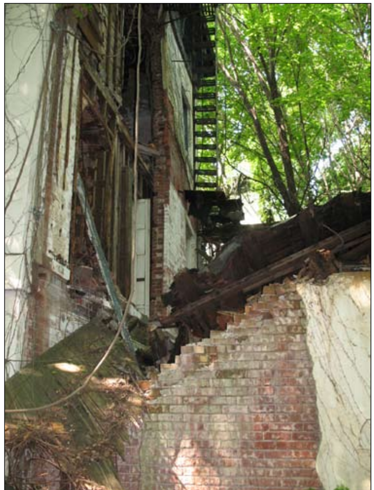
Collapsed 20th century rear addition 6
