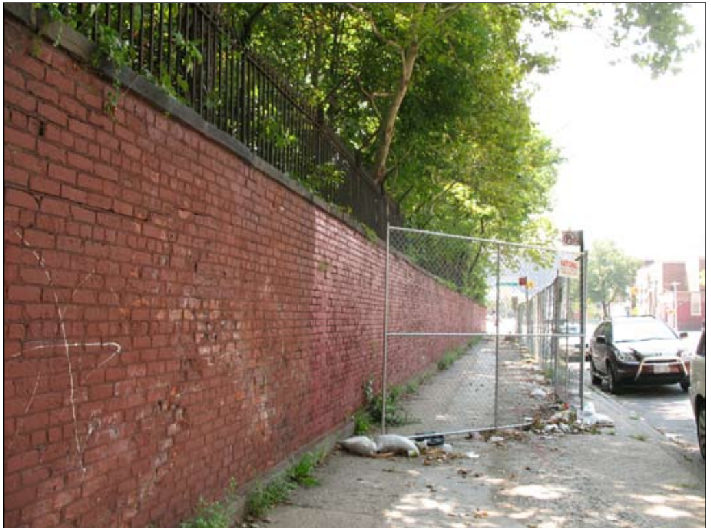
View south on Navy Street. The brick wall and iron fence that borders Admirals Row is on the left. The chain link fence on the sidewalk prohibits pedestrian access on the sidewalk by the Timber Shed, which has been determined to be structurally unsound 20
