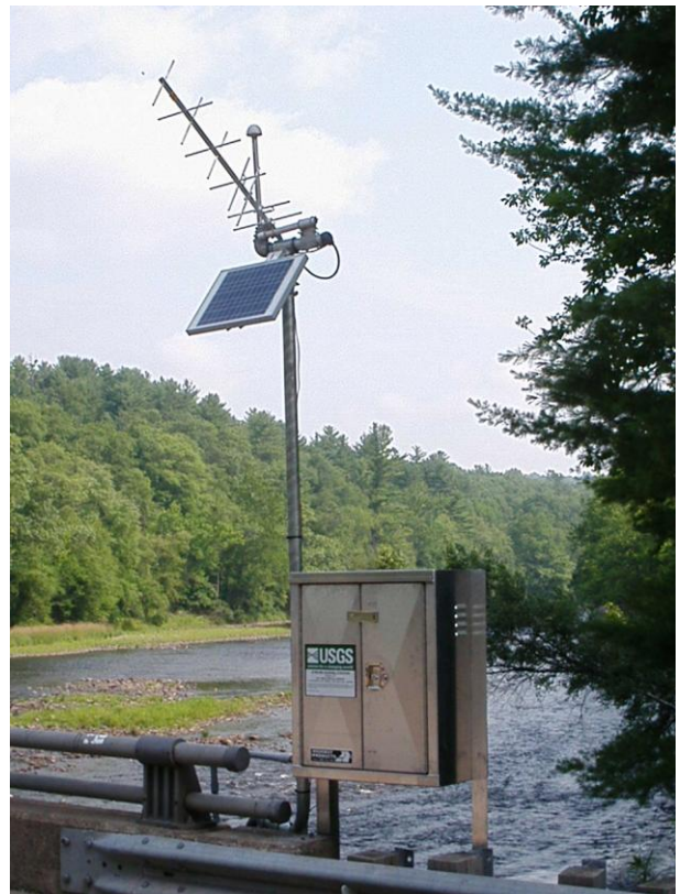
USGS stream gage provides reliable, real-time flow measurements.
