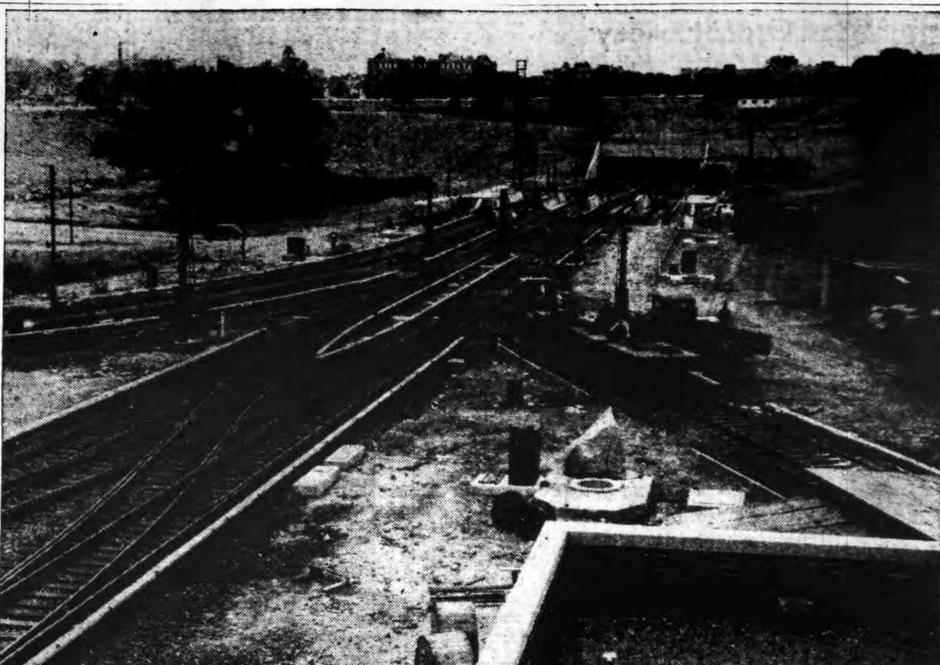
The yards of the new subway in Kew Gardens nears completion. Most of the remaining work is the installation of cables, wiring and lighting. The picture shows the entrance to the yards from the subway tunnel just north of Queens boulevard, as seen from the control tower building.
