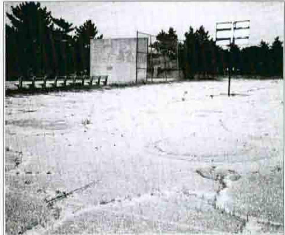
Figure 56: Deteriorating game court surfaces
