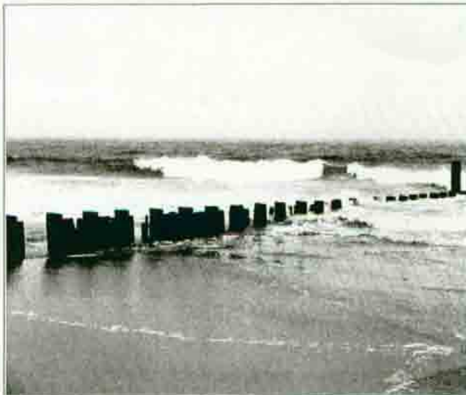
Figure 68: Typical deteriorated jetty
