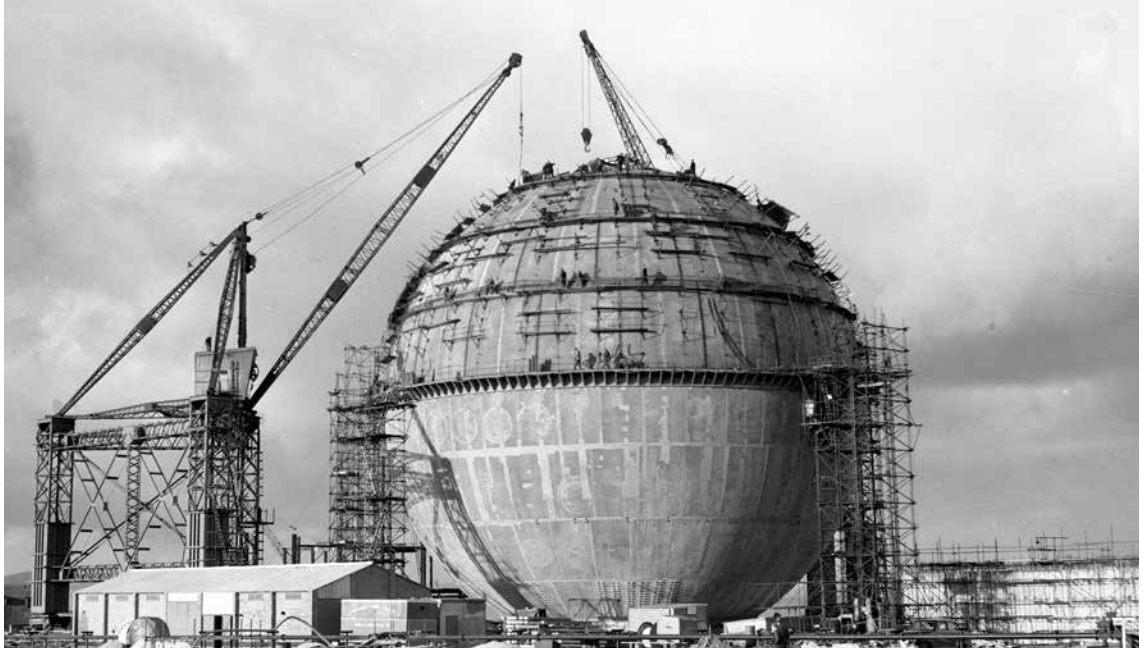
Construction of the Dounraey Fast Reactor sphere, by Motherwell Bridge & Engineering Company Ltd., Caithness, 1956. © Nuclear Decommissioning Authority & Dounraey Site Restoration.'
