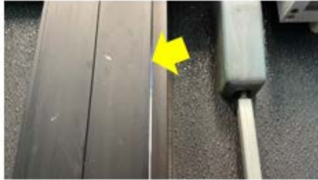
Caulking – gaps at door assembly are allowing unwanted air leakage as seen by clear daylight between trim (Alexander D Sullivan School).
