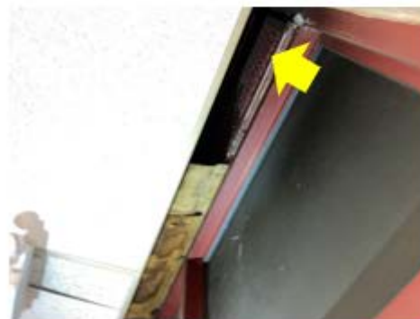
Wall Air Sealing – the air barrier is not continuous at the exterior wall; a louver over the door is stuck open resulting in excessive air leakage into the building (Joseph Brensinger School).
