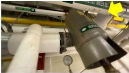
Tank Insulation – the un-insulated air separator tank needs to be insulated to reduce heating distribution losses (Dr Maya Angelou School).
