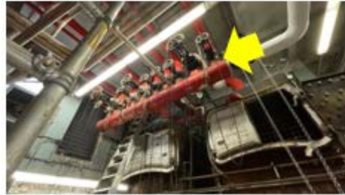
Valve & Fitting Insulation – bonnets should be insulated with removable blankets to limit heat loss at otherwise well insulated steam gate valves (Charles Tefft School)
