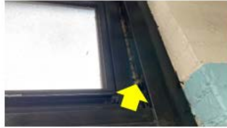
Caulking – dirty fiberglass is a clear sign of air leakage behind the snap trim of the window, caulk needs to be applied to the window assembly to reduce air leakage (Alexander D Sullivan School).
