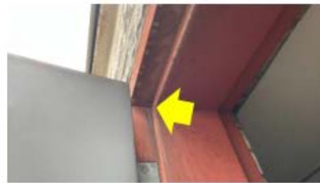
Door Weather Stripping – damaged/missing weather stripping needs to be replaced to reduce drafts and air leakage at the door assembly (Michael Conti School).
