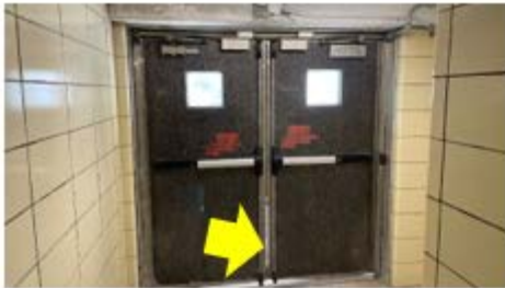
Door Weather Stripping – daylight at the center and bottom of the door shows clear envelope weaknesses that need to be addressed with improved weather stripping (Academy 1 MS).
