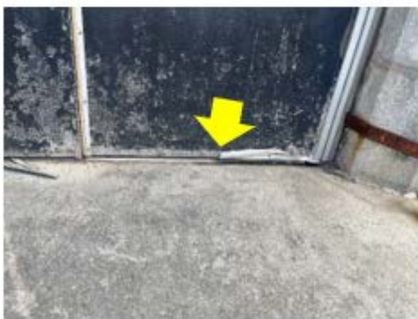
Door Weather Stripping – damaged/missing weather stripping needs to be replaced to reduce drafts and air leakage at the door assembly (Mahatma Gandhi School).
