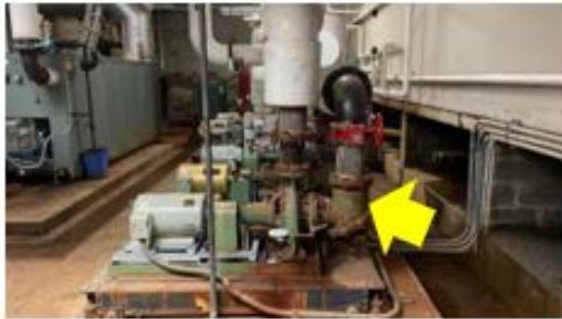
Valve & Fitting Insulation – components at the pump station need to be insulated to reduce unnecessary distribution losses (Ronald McNair School).
