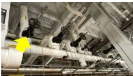
Valve & Fitting Insulation – bonnets should be insulated with removable blankets to limit heat loss at otherwise well insulated steam gate valves (William Dickinson School).
