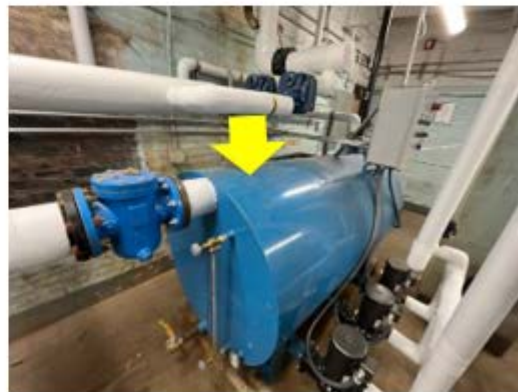
Tank Insulation – the condensate tank represents a large surface area in the heating distribution system that needs to be insulated to improve efficiency (Mahatma Gandhi School).
