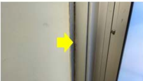
Caulking – gaps between the window trim pieces are building up with dust/debris as air leaks into and out of the building (Glenn D Cunningham Center).
