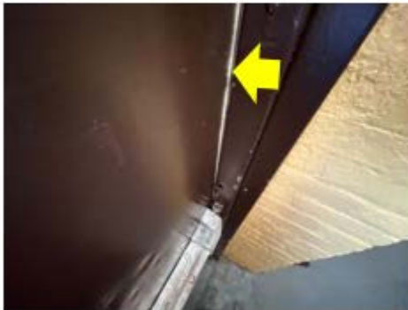
Door Weather Stripping – daylight at the sides of the door shows clear envelope weaknesses that need to be addressed with improved weather stripping (Anthony J Infante School).
