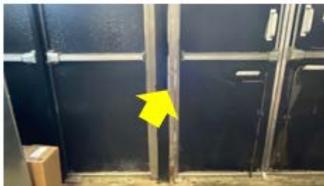
Door Weather Stripping – daylight at the door shows clear envelope weaknesses that need to be addressed with improved weather stripping (James J Ferris School).
