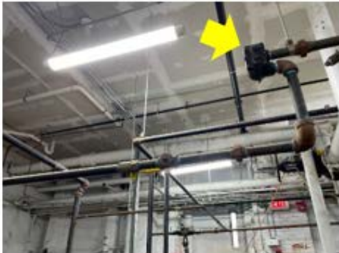
Valve & Fitting Insulation – the steam trap and surrounding pipes are not insulated which is leading to unnecessary distribution losses (Danforth ECC).
