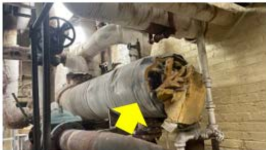
Tank Insulation – damaged insulation should be removed and replaced to reduce unnecessary heating distribution losses (Lincoln HS).
