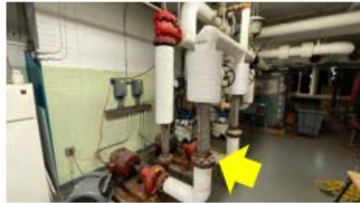
Valve & Fitting Insulation – components at the pump station need to be insulated to reduce unnecessary distribution losses (JwLK School).
