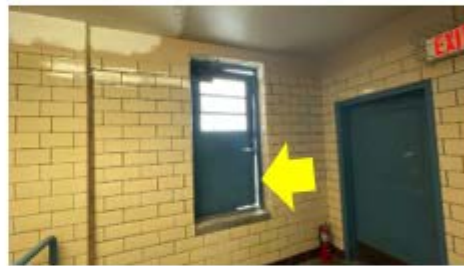
Door Weather Stripping – daylight at the side and bottom of the door shows clear envelope weaknesses that need to be addressed with improved weather stripping (Charles T. DeLury School).
