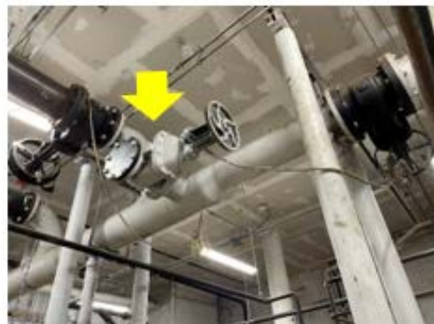
Valve & Fitting Insulation – the valves are not insulated which is leading to unnecessary distribution losses (Danforth ECC).
