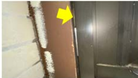
Caulking – gaps between the window frame and block wall are a direct pathway between interior and exterior of the building resulting in air leakage (Danforth ECC).
