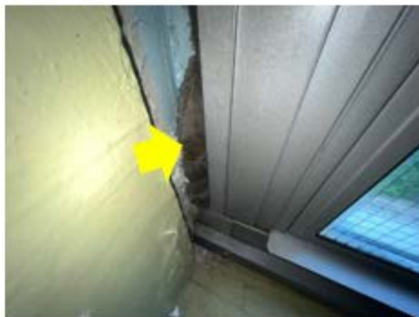
Caulking – dirty fiberglass is a clear sign of air leakage behind the snap trim of the window, caulk needs to be applied to the window assembly to reduce air leakage (St. Anthony, Clarendon School).
