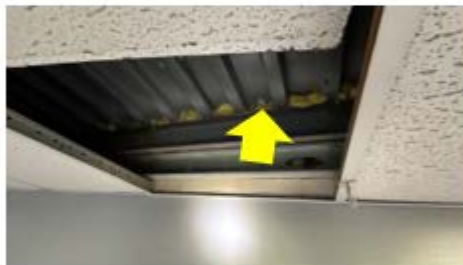
Roof-Wall Intersection Air Sealing – air permeable fiberglass installed in the roof-wall intersection is allowing air infiltration and exfiltration (Alfred Zampella School).
