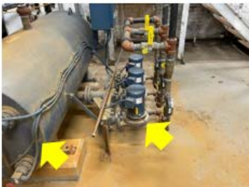
Tank Insulation – the condensate tank and surrounding pipes represents a large surface area in the heating distribution system that needs to be insulated to improve efficiency (Danforth ECC).
