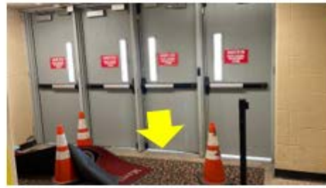
Door Weather Stripping – daylight at the door shows clear envelope weaknesses that need to be addressed with improved weather stripping (Fred Martin School).
