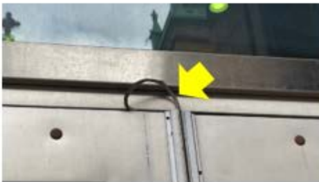
Door Weather Stripping – damaged/missing weather stripping needs to be replaced to reduce drafts and air leakage at the door assembly (Christa McAuliffe).
