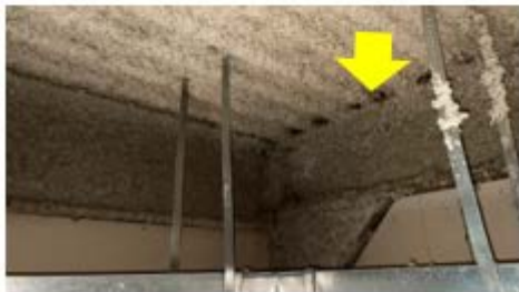
Roof-Wall Intersection Air Sealing – gaps in fireproofing spray are bulging up with dust/debris; a clear sign of air leakage through the roof-wall intersection of the building (President Barack Obama School).
