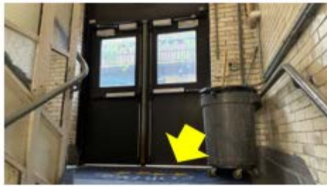
Door Weather Stripping – daylight at the bottom of the double door assembly is a clear sign of air leakage that can be eliminated by installing proper weather stripping (Rafael Cordero School).
