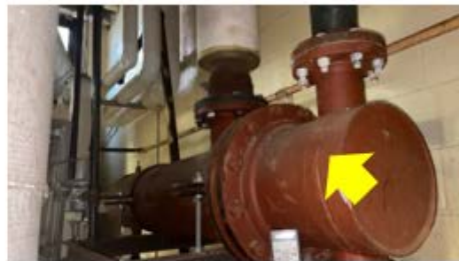
Tank Insulation – the un-insulated heat exchanger needs to be insulated to reduce heating distribution losses (Lincoln HS).
