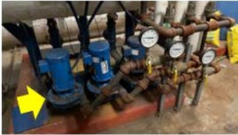
Valve & Fitting Insulation – condensate pumps and pipe attached to the condensate tank should be insulated to reduce heating distribution losses (Alexander Sullivan School).
