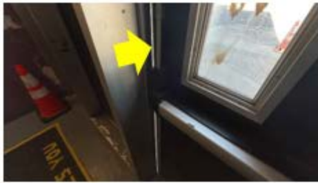
Door Weather Stripping – daylight at the door shows clear envelope weaknesses that need to be addressed with improved weather stripping (Ezra Nolan School).
