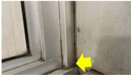
Caulking – gaps between the window snap trim is partially caulked, sealants should be applied at all trim intersections to reduce air leakage (Ezra L Nolan School).
