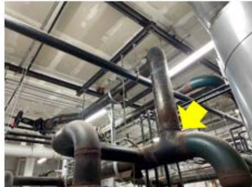
Valve & Fitting Insulation – pipes are not insulated which is leading to unnecessary distribution losses (Danforth ECC).
