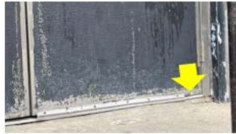
Door Weather Stripping – damaged/missing weather stripping needs to be replaced to reduce drafts and air leakage at the door assembly (Alfred Zampella).
