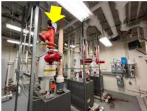
Valve & Fitting Insulation – the strainer and pump are not insulated which is leading to unnecessary distribution losses (Patricia Noonan School).
