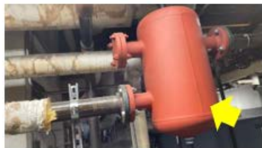
Tank Insulation – the un-insulated air separator tank needs to be insulated to reduce heating distribution losses (Fred Martin School).
