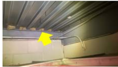
Roof-Wall Intersection Air Sealing – air permeable fiberglass installed in the roof-wall intersection is allowing air infiltration and exfiltration (Christa McAuliffe School).
