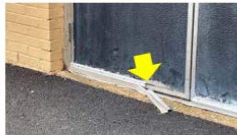
Door Weather Stripping – damaged/missing weather stripping needs to be replaced to reduce drafts and air leakage at the door assembly (James J Ferris School).
