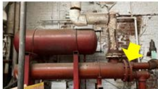
Tank Insulation – the un-insulated heat exchanger needs to be insulated to reduce heating distribution losses (Rafael Cordero).
