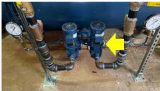
Valve & Fitting Insulation – condensate pumps and pipe attached to the condensate tank should be insulated to reduce heating distribution losses (Jotham Wakeman School).
