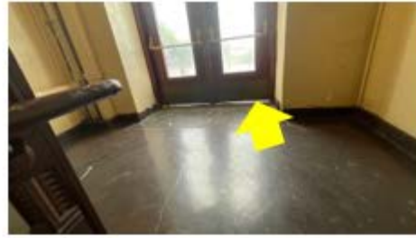
Door Weather Stripping – daylight at the bottom of the double door assembly is a clear sign of air leakage that can be eliminated by installing proper weather stripping (William Dickinson School).
