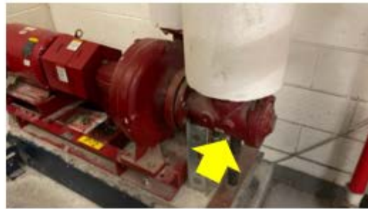
Valve & Fitting Insulation – components at the pump station need to be insulated to reduce unnecessary distribution losses (Dr Maya Angelou School).
