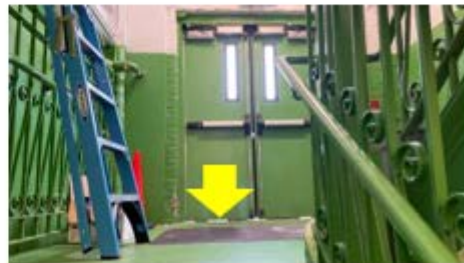
Door Weather Stripping – daylight at the center and bottom of the door shows clear envelope weaknesses that need to be addressed with improved weather stripping (Danforth ECC).
