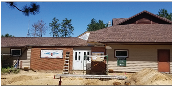
Blue Wing Village family/community center being renovated to make the main entrance safe for elders and physically disabled.
