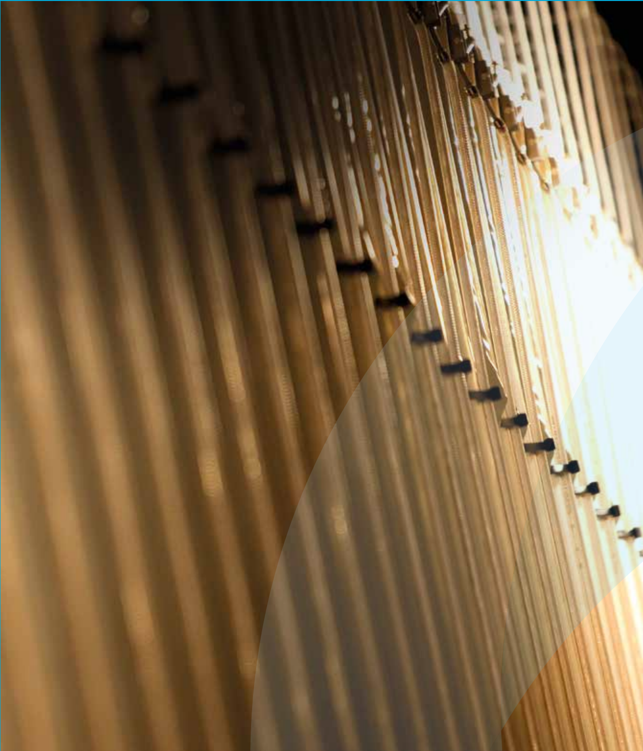
Inside a URENCO centrifuge hall.
