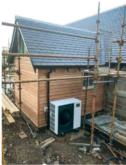
An air source heat pump fitted outside an Ecology-backed energy efficient self-build in Scotland
