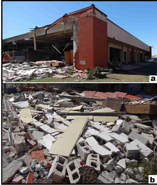
Figure 15. Damage to a concrete framed building at the Canadian Valley Technology Center: a) collapse of concrete masonry walls, b) closer view showing the absence of vertical steel reinforcement in the wall. Damage to this building was rated EF2.
