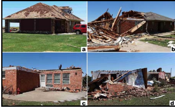
Figure 12. Increasing damage ratings to wood-framed houses: a) EF0, b) EF1, c) EF2, and d) EF3.
