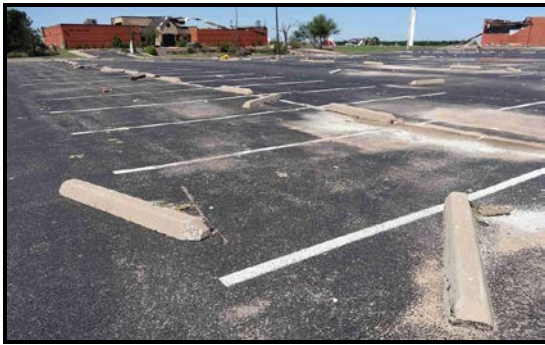
Figure 22. Westward movement of parking stops at the Vo-Tech Center. Such movement occurred in between buildings rated EF1 and EF2.
