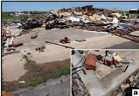
Figure 13. All walls on this home had collapsed in the center of the tornado path. Close examination revealed no nuts or washers on the anchor bolts (inset a). Therefore, a rating of EF3 was assigned instead of EF4.
