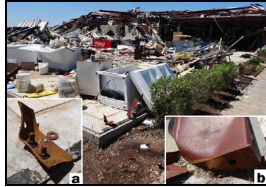
Figure 17. Destruction of a metal building at the Oklahoma West Livestock Market. Steel column base plates were: a) torn along welded connections, or b) pulled through their anchor bolts. Damage to this building was rated EF3.
