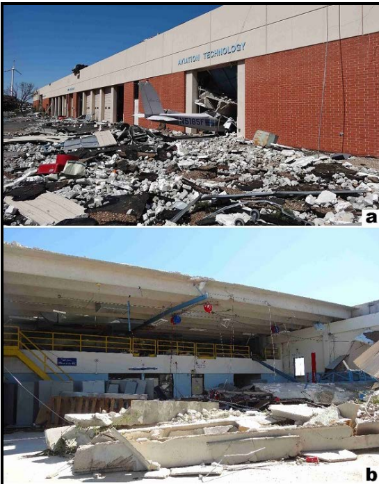
Figure 16. Damage to the Aviation Technology Department at the Canadian Valley Technology Center: a) an airplane in the doorway and b) collapsed large span, steel-reinforced concrete double tee roof beams. The beams fractured at midspan due to wind uplift forces. Damage to this building was rated EF3.
