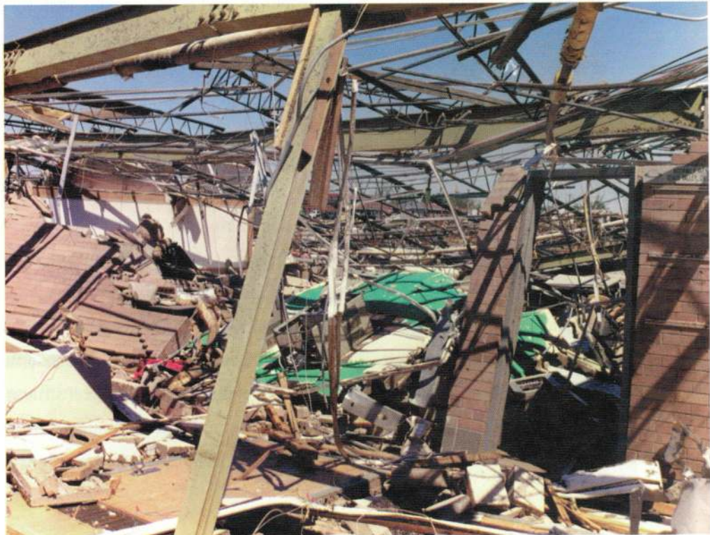
FIGURE 22. KELLY ELEMENTARY SCHOOL, MOORE, OK
