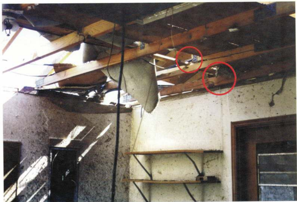
FIGURE 5. FAILURE AT KNOTS IN WOOD MEMBERS
