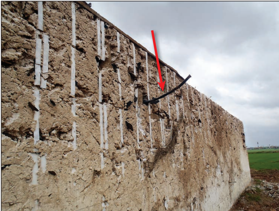
Figure 7. Observation 5: ICF structure penetrated by metal wind-borne debris elements (Newcastle, OK)
