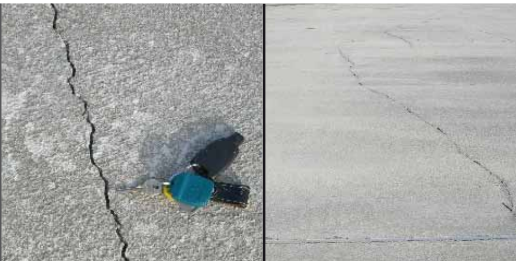
photo 16 Cracking in concrete
