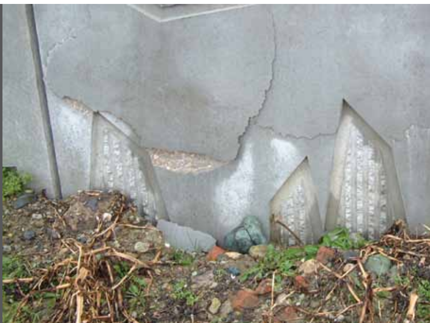
photo 14 Deterioration due to freezing
