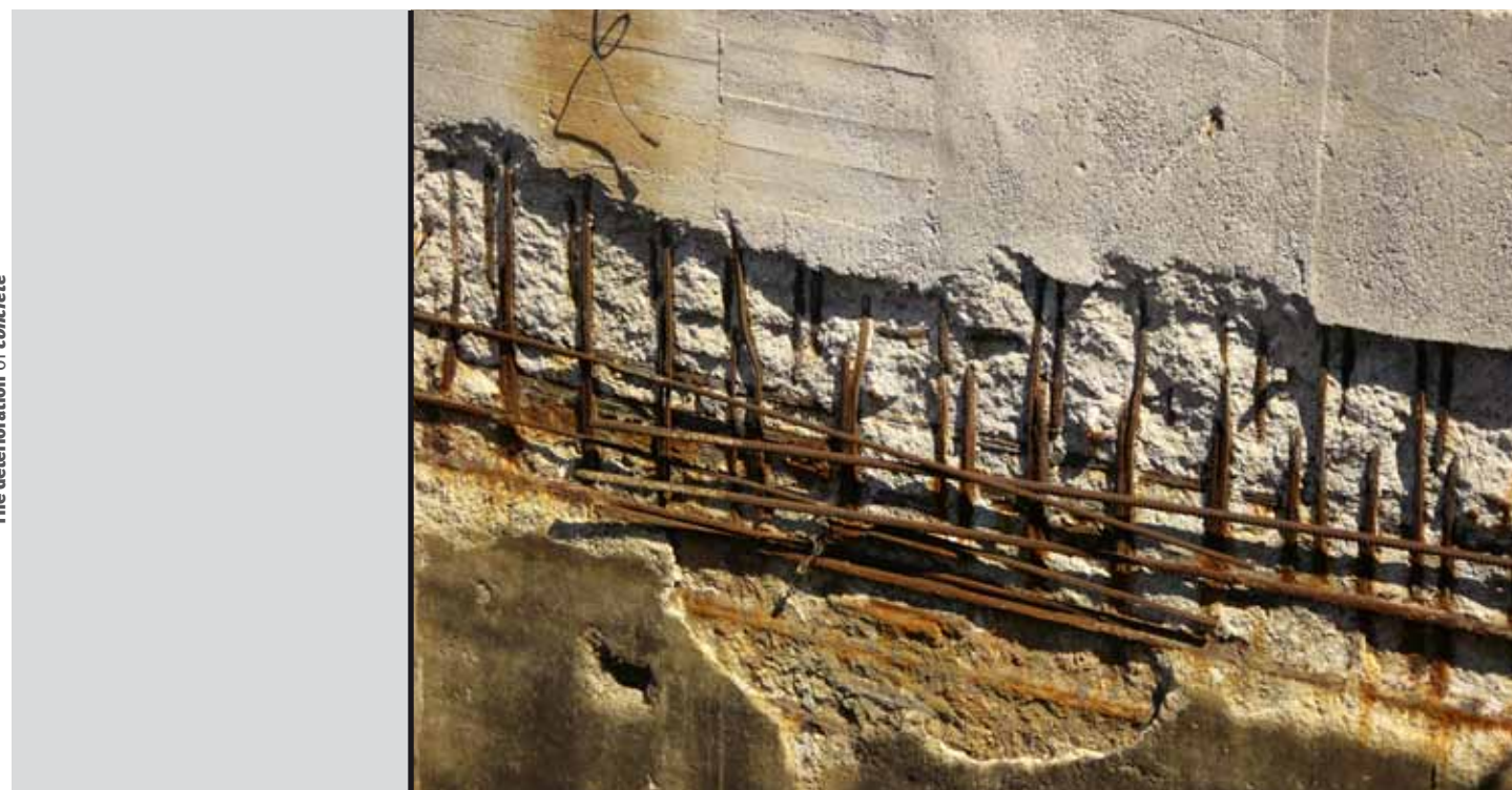
The deterioration of concrete
