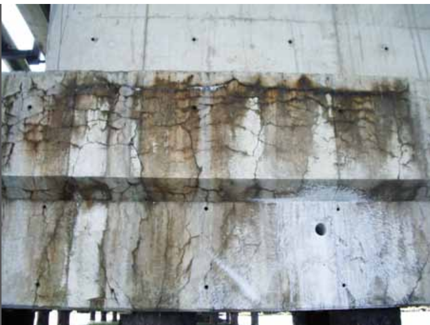
photo 11 Deterioration due to alkali- aggregates reaction
