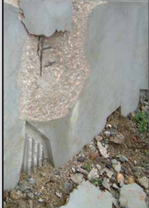
photo 15 Deterioration due to freezing
