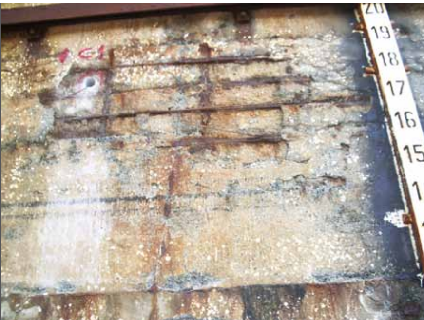
photo 10 Corrosion caused by chloride attack
