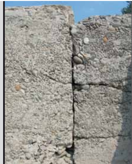
photo 18 An example of erosion
