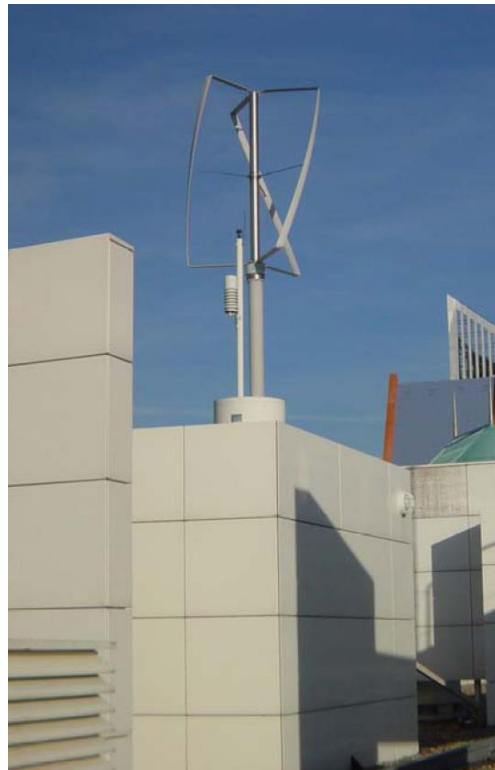
Figure 23. Turby triple blade wind turbine design on top of a building.
