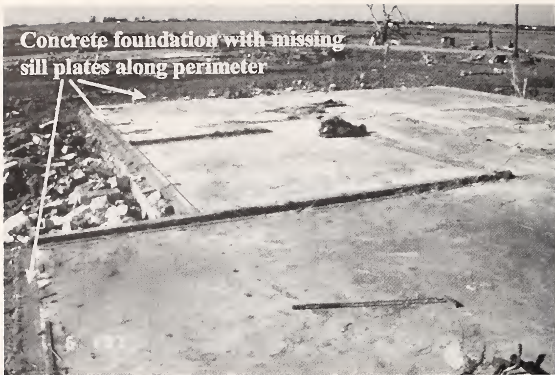
Figure 11. Close-up view of a typical slab-on-grade foundation of houses in the Double Creek Estates subdivision. Only one sill plate remains connected to the concrete foundation.
