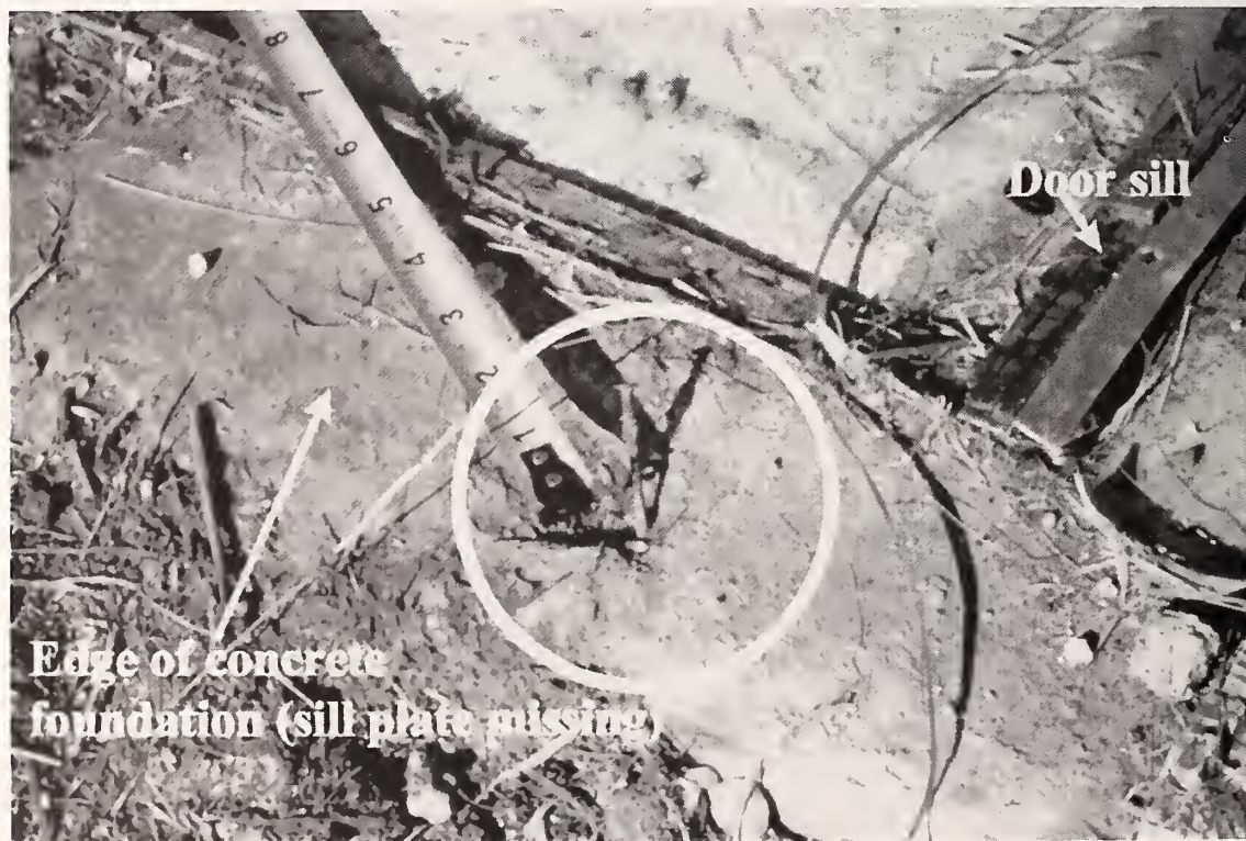
Figure 12. Evidence of nail that was used for connecting sill plate to concrete foundation.
