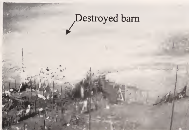
Figure 9. Destroyed barn located between culvert plant complex and Double Creek Estates subdivision.
