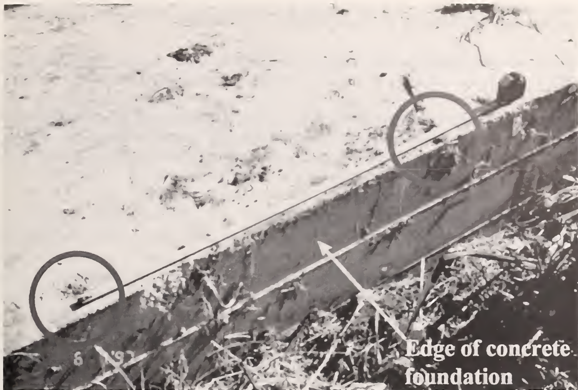
Figure 13. Evidence of pullout of nails used to fasten sill plates to concrete foundation.
