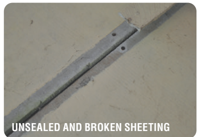
BROKEN ASBESTOS CEMENT SHEETING
