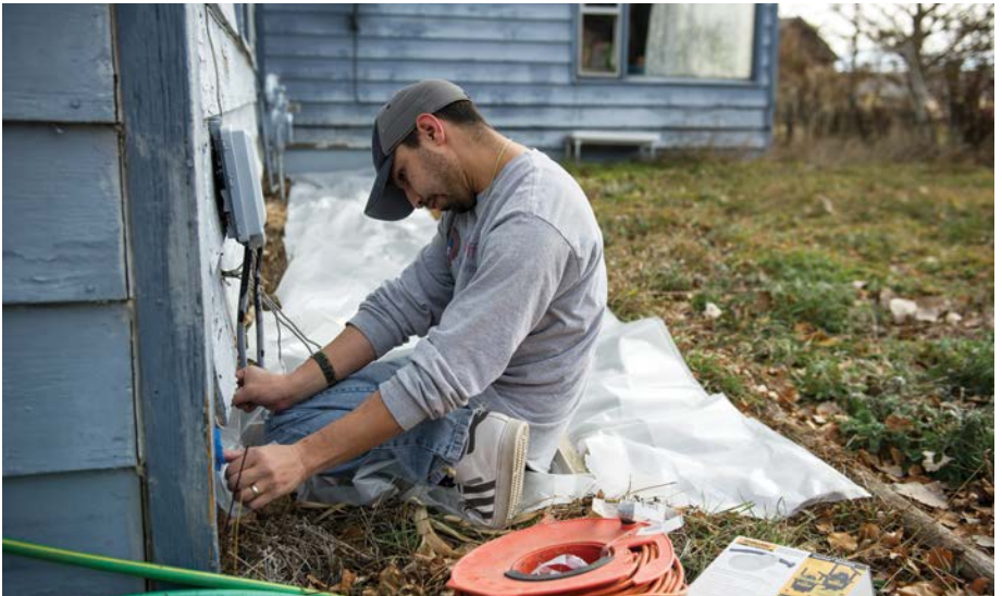
Weatherization can reduce energy bills and improve the efficiency, health, and safety of the home.
