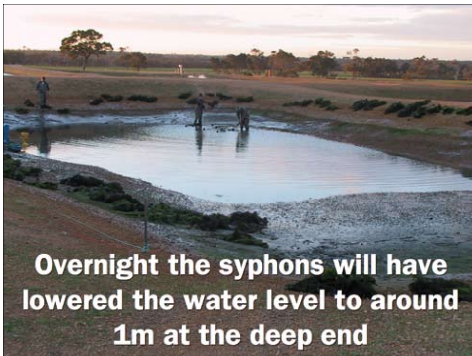
Slide 33. Overnight the syphons will have lowered the water level to around 1m at the deep end.
