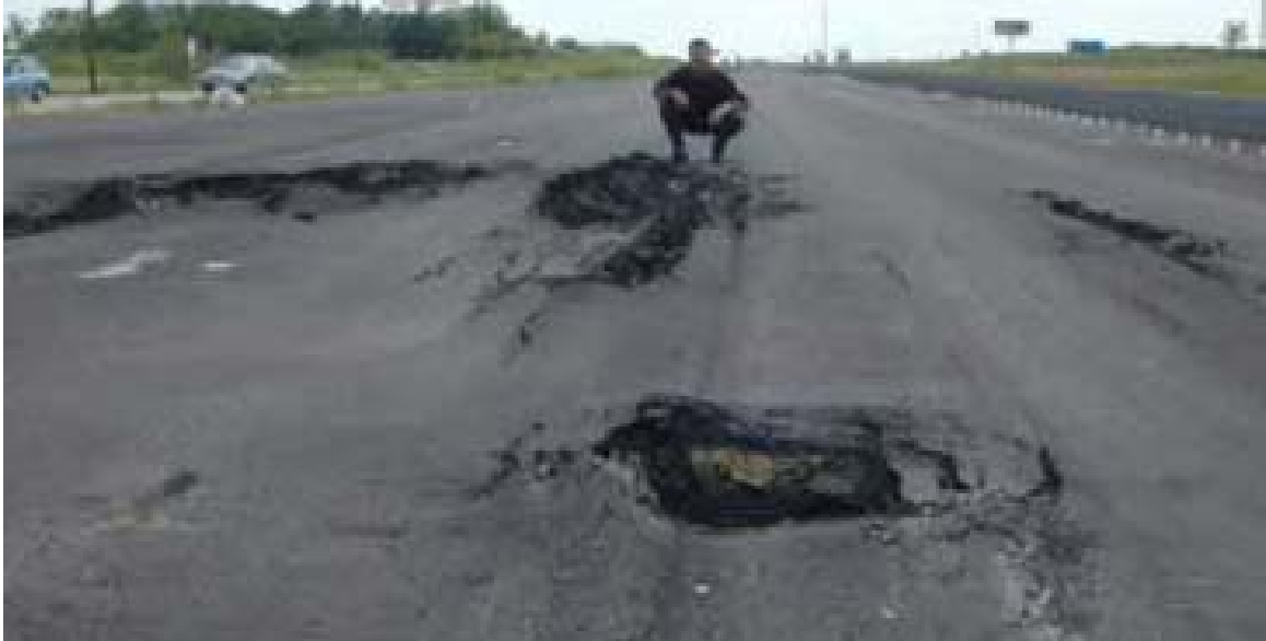
Figure 1: Extreme example of pavement failure from unstable soils
