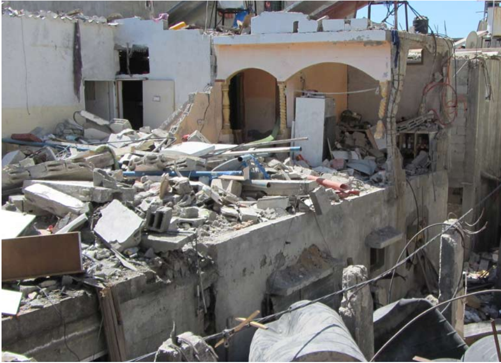
The ruins of the al-Bayumi family home. Photo: Khaled al-'Azayzeh, B'Tselem, 27 Aug. 2014.
