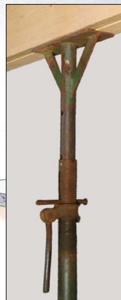
Long post-shore jacks are useful for several of these suggested stiffening strategies. They vary in price, depending on lifting capacity; prices start around $25 apiece ( www.ablebuilders.com ).
