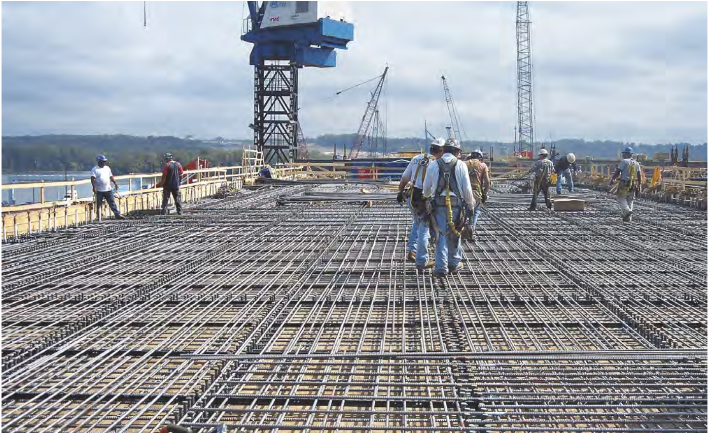
Installation of duplex stainless steel rebar on a large bridge deck. © Hardesty & Hanover, LLP
