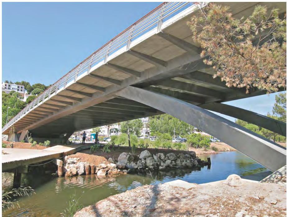
Bridge in Cala Galdana on Menorca fabricated using 2205 duplex stainless steel. © PEDELTA
