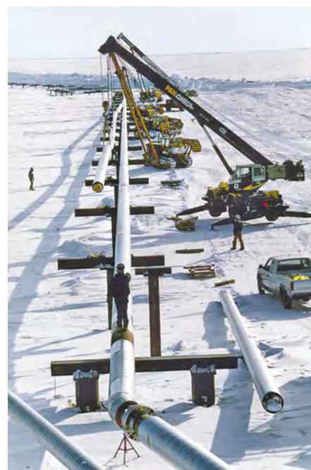
Installation of insulated 24 inch 2205 pipe on vertical support members in Prudhoe Bay. © Arco Exploration and Production Technology
