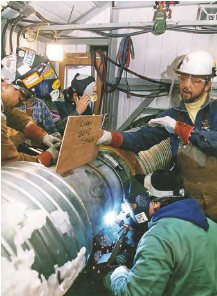
Mechanized welding of large diameter duplex stainless steel cross-country pipeline. © Arco Exploration and Production Technology
