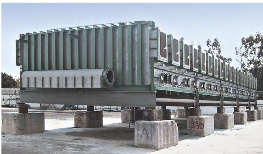
Multi stage flash seawater desalination unit constructed of S32101 and 2205 duplex stainless steels. © Outokumpu
