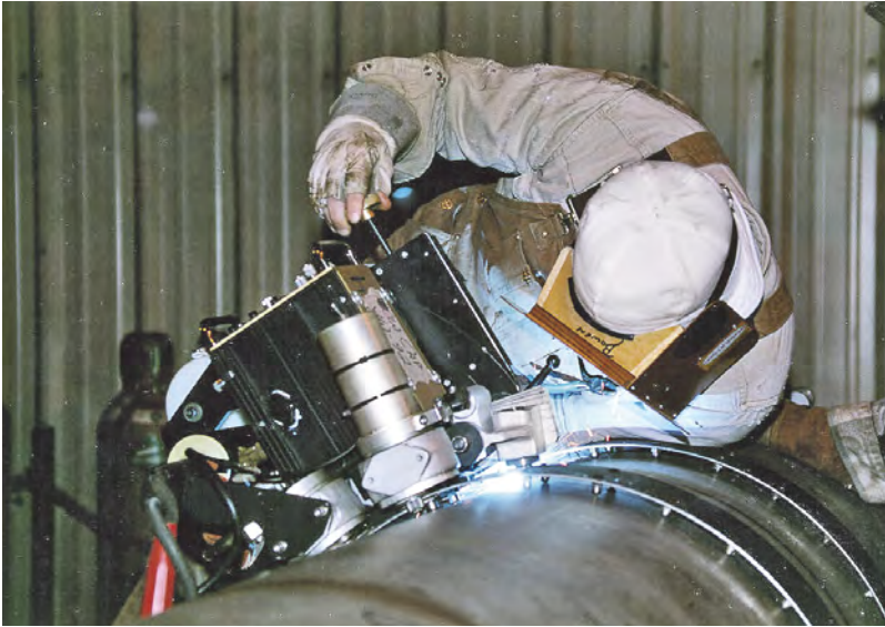
Mechanized welding of large diameter duplex stainless steel pipeline on Alaska's north slope. © Arco Exploration and Production Technology
