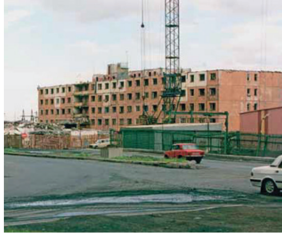
Damage associated with permafrost deterioration necessitates the demolition of a nine-story residential building in Norilsk that had only been in use for 21 years (July 2001).
