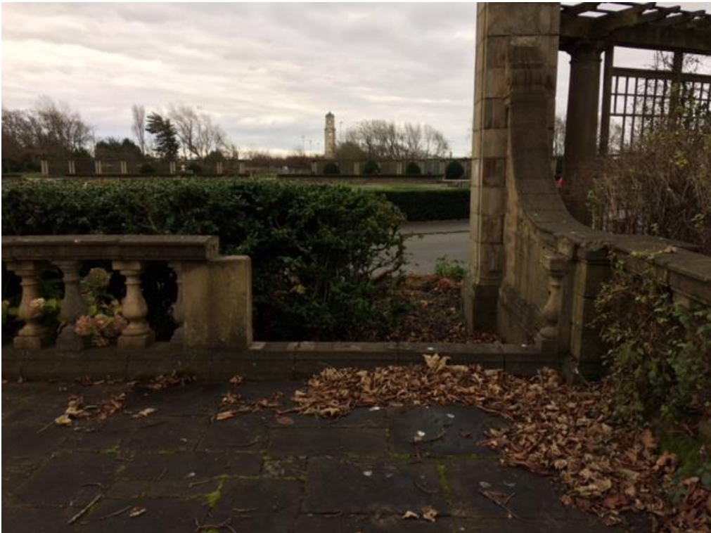
Missing balustrade on café terrace
