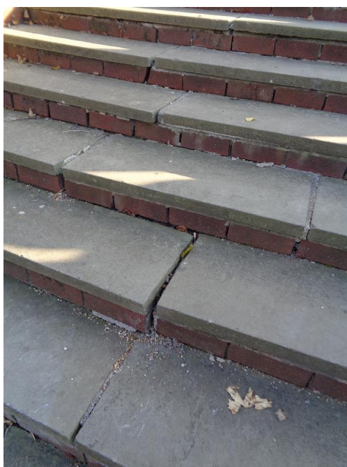
Steps down from Italian Garden in need of repair (recently repaired and re-opened to public)
