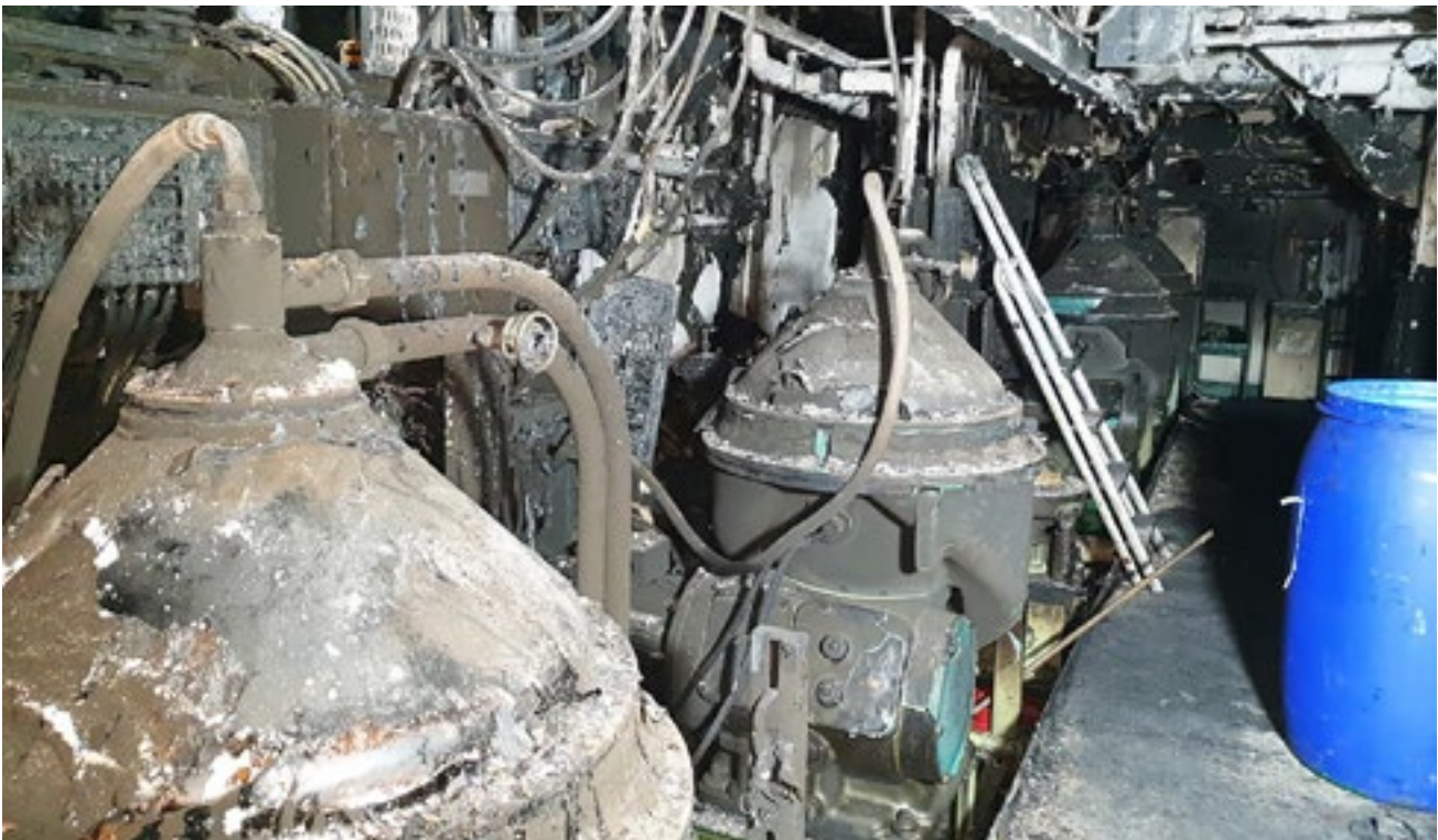
Figure 1: Fire-damaged fuel purifier room
