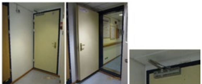
Fire Doors and Closing Mechanism
