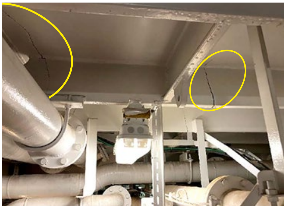
Figure 2: Cracks in the supporting steelwork
