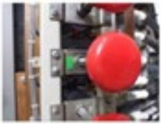
Battery disconnect switch
