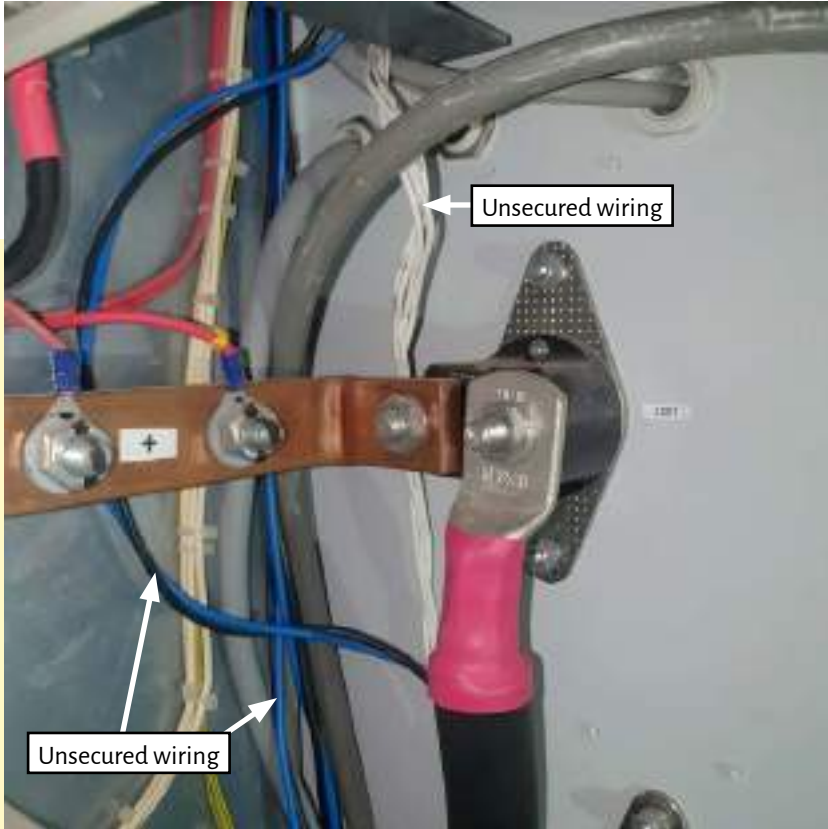
Figure 2: Unsecured wiring in the electrical control panel
