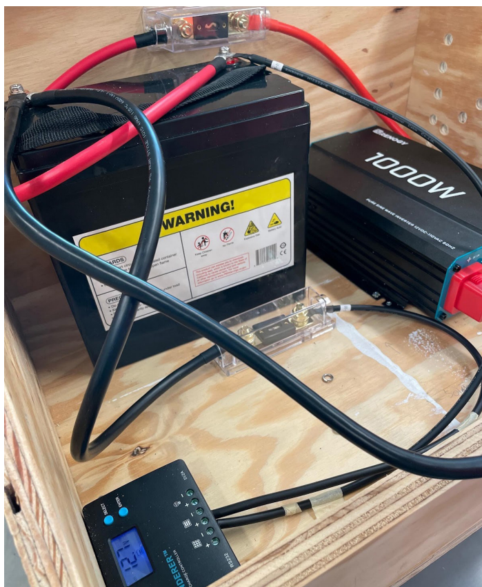
The wiring of the electronics box
