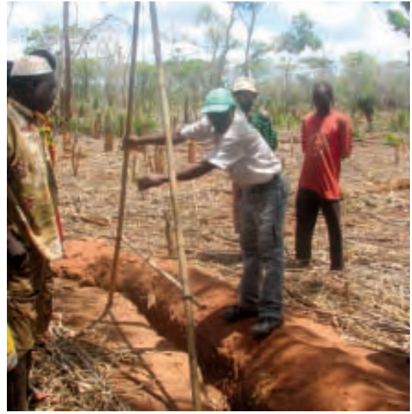
Laying out contour ditches in Quirimbas National Park, Mozambique. The ditches capture runoff during storms, increasing soil moisture and reducing soil erosion, so crop yields increase.
