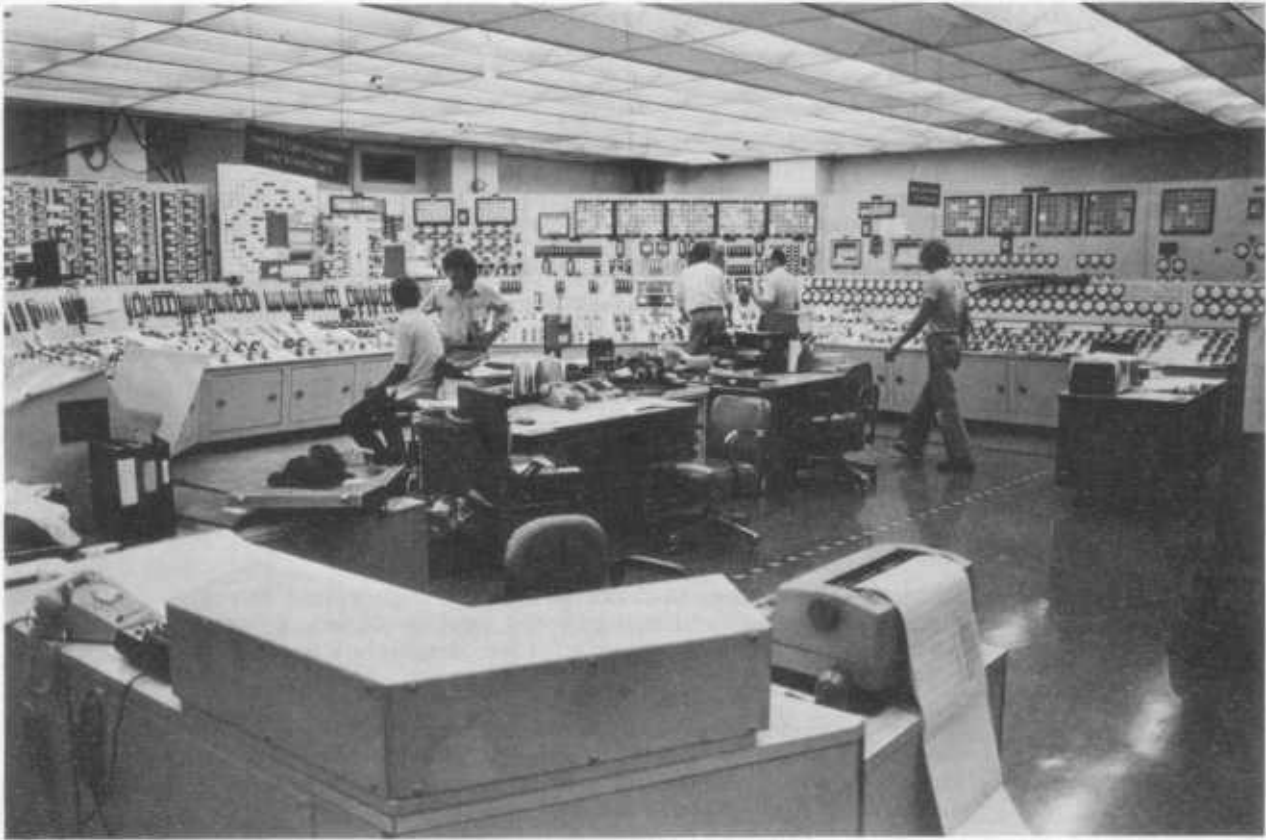
FIGURE 11-48. TMI Control Room (Postaccident)
