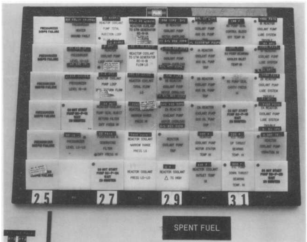
FIGURE 11-53. Typical TMI-2 Alarm Panel
