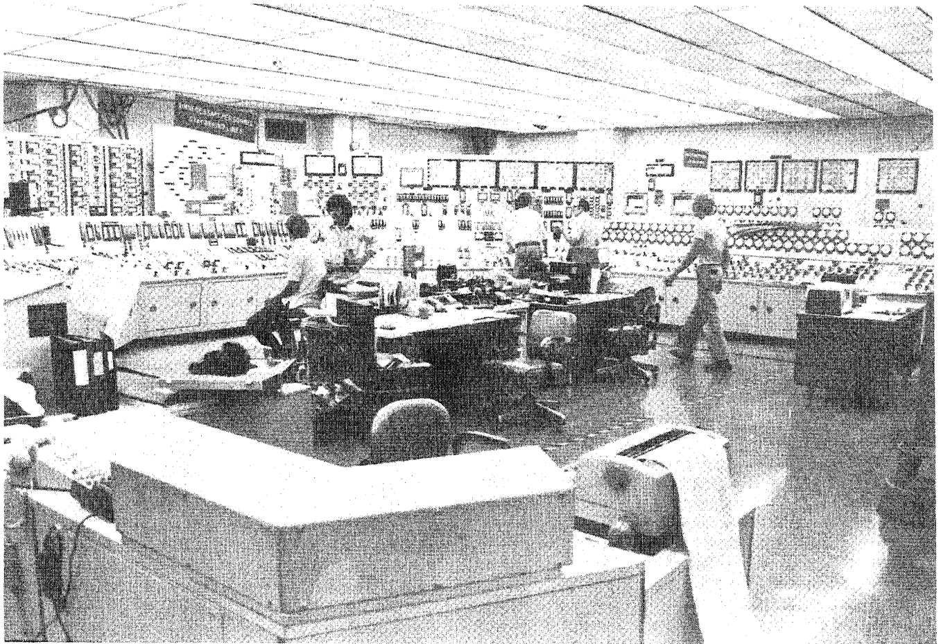
The control room for TMI Unit 2 is shown above. The instruments and controls are deployed in a U-shaped pattern in a design intended to permit one operator to supervise operations under nor-
