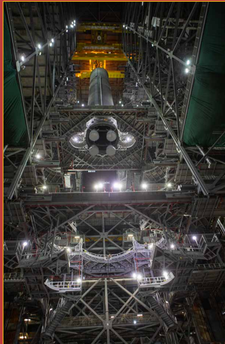
In this view looking up inside the Vehicle Assembly Building at NASA's Kennedy Space Center, workers use a crane to lower the Space Launch System Core Stage pathfinder into High Bay 3 on Oct. 16, 2019. Photo credit: NASA/Ben Smegelsky
