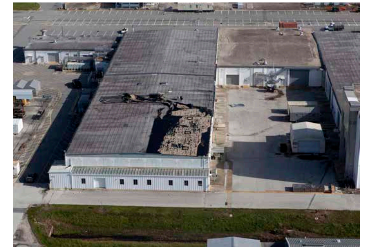
An industrial building behind the Space Station Processing Facility shows some roof damage following Hurricane Irma. Photo credit: NASA/Bill White
