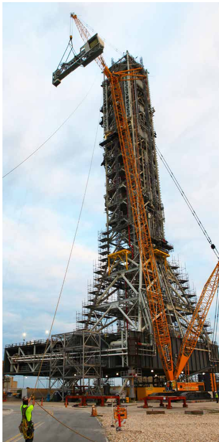
A crane positions the Orion crew access arm so it can be attached to the mobile launcher (ML). The arm will be installed at about the 274-foot level on the 380-foot-tall ML tower. Photo credit: NASA/Bill White
