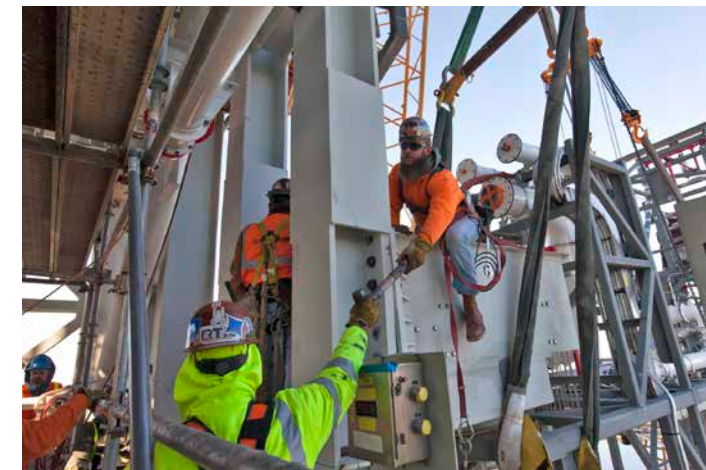
Construction workers with JP Donovan install the Interim Cryogenic Propulsion Stage Umbilical (ICPSU) to the tower of the mobile launcher at about the 240-foot-level on March 16, 2018. The last of the large umbilicals to be installed on the tower, the ICPSU will provide super-cooled hydrogen and liquid oxygen to the Space Launch System rocket's interim cryogenic propulsion stage, or upper stage, at T-0 for Exploration Mission-1. Photo credit: NASA/Ben Smegelsky
