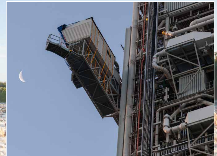
In this view, Exploration Ground Systems' mobile launcher's crew access arm (CAA) can be seen. The CAA will interface with the agency's Space Launch System (SLS) rocket at the Orion crew hatch, providing entry and exit from the Orion crew module. The first crewed flight aboard Orion will be Artemis 2, after the uncrewed Artemis 1 launch verifies SLS and Orion as an integrated system. Photo credit: NASA/Ben Smegelsky
