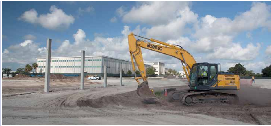
At the construction site for the new, modernized Central Campus Headquarters building at NASA's Kennedy Space Center, concrete pilings have been driven into the ground at varying depths as a test. A bulldozer is clearing the site on May 14, 2015 for more pilings to be added. In the background is the existing Headquarters Building. Photo credit: NASA
