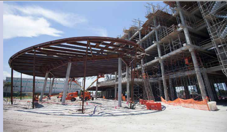
Left: Construction was in full swing on the new Central Campus Headquarters building on July 11, 2016 at NASA's Kennedy Space Center. Photo credit: NASA/Ben Smegelsky
