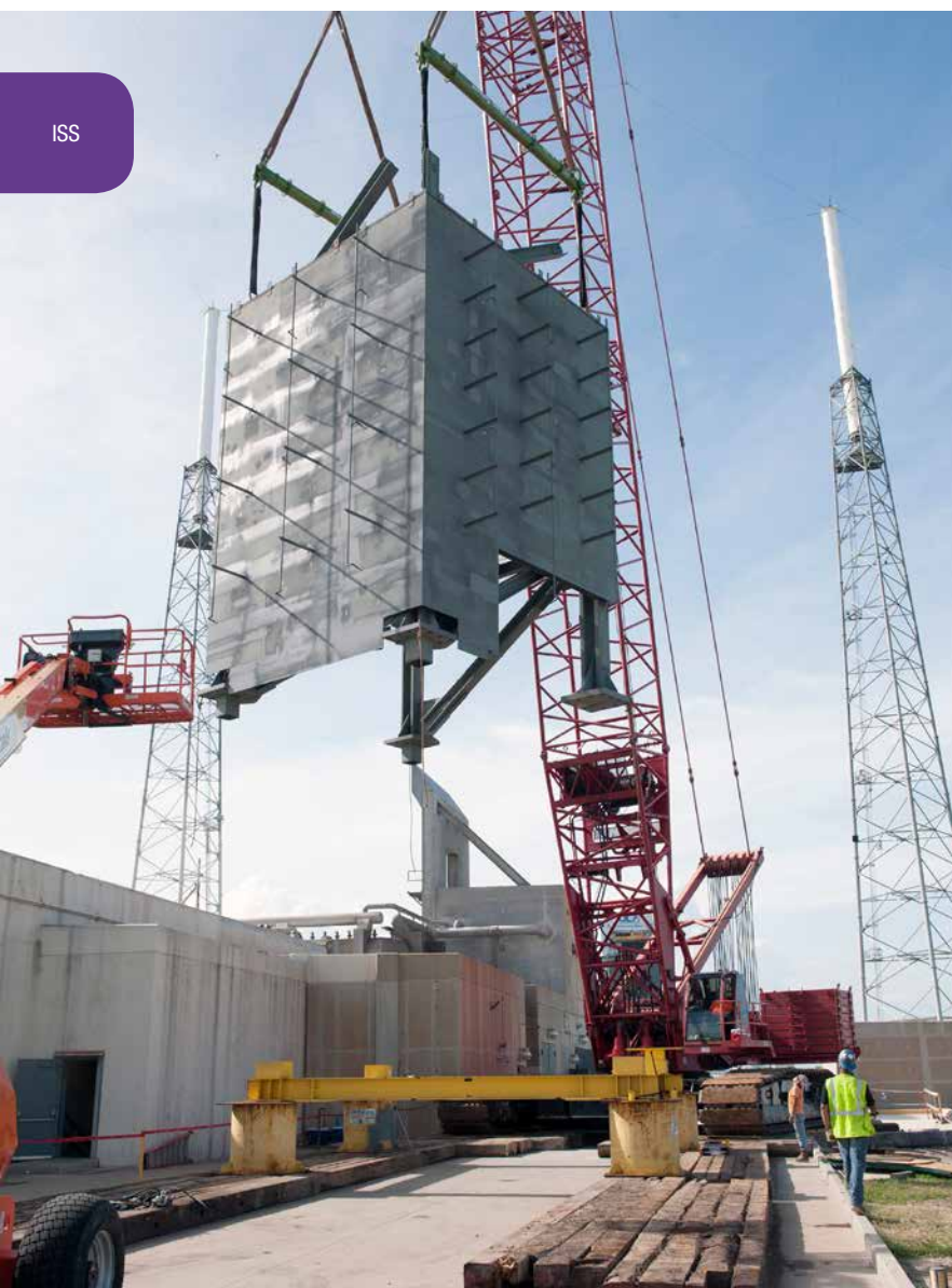
A crane lifts the first tier for placement at Space Launch Complex-41 at Cape Canaveral Air Force Station, Florida, to form the Crew Access Tower under construction by Boeing and United Launch Alliance. The steel structure is being built in seven pieces that will be stacked atop each other to form a 200-foot-tall tower complete with elevator, communications and power infrastructure, and an escape system. The tower will provide astronauts and ground support teams access to Boeing's CST-100 Starliner spacecraft, in development in partnership with NASA's Commercial Crew Program. Photo credit: NASA/Tony Gray
