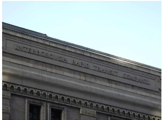
IRT Powerhouse, terra cotta nameplate detail at the top of the eastern façade, December 3, 2011.
