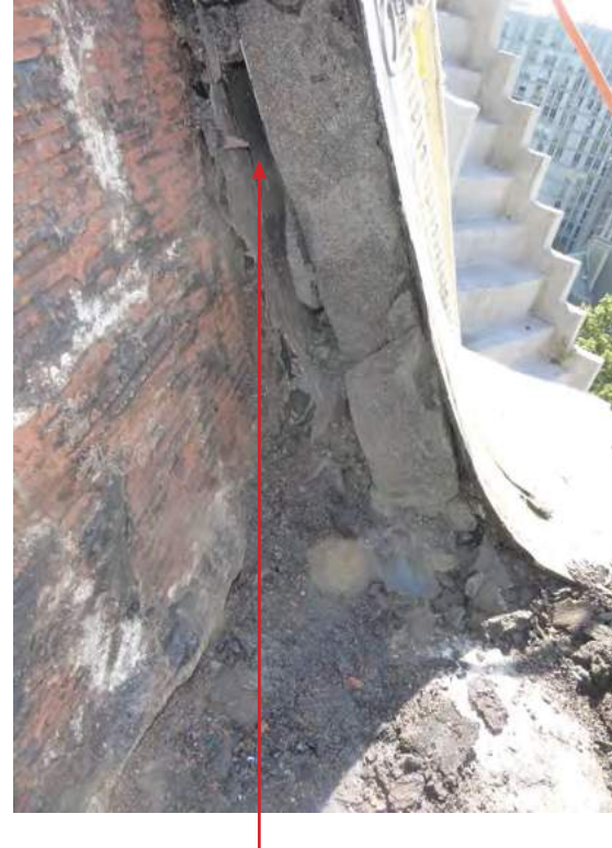
Large gap between Foam-glass Insulation and Tile Dome
