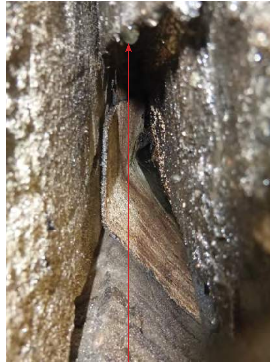
Water droplets on original waterproofing membrane
