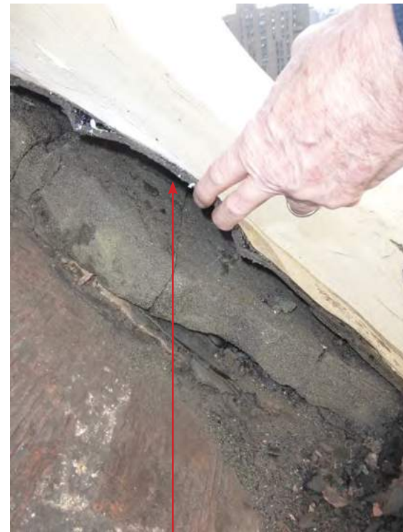
Outer waterproofing membrane is not adhered to Foamglass Insulation
