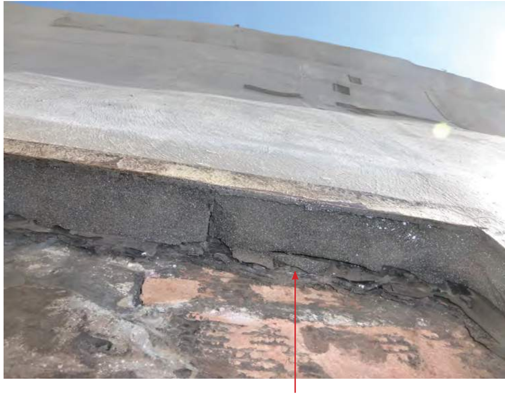
Dry and crumbly consistency of the original membrane
