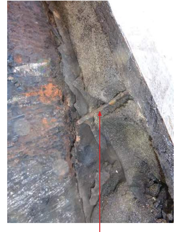
Advanced Corrosion at screws (mechanical fasteners for insulation)
