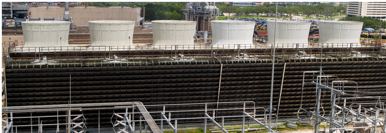
Figure 11.2 A mechanical-draft cooling tower. The fans are located within the cylindrical housings at the top. Air is drawn in through the louvers on the side.
