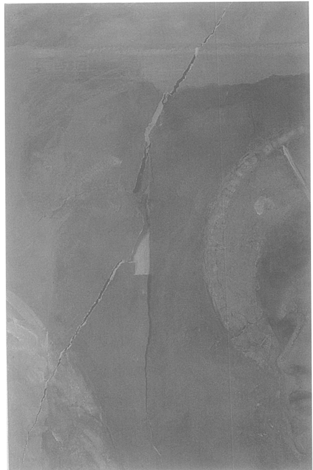
Fig. 9. Law detail of top left showing new damage caused by the mounting system
