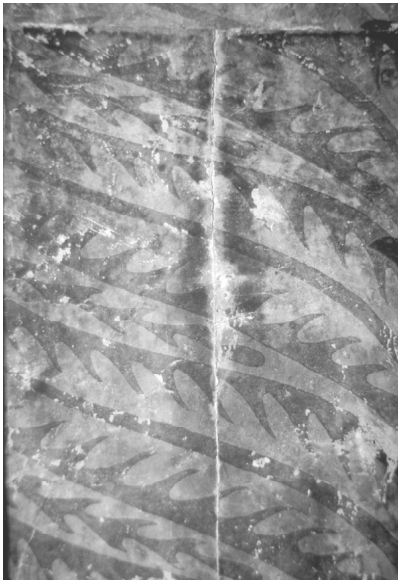
Fig. 12.. Cecil Hall, detail: stained area before treatment
