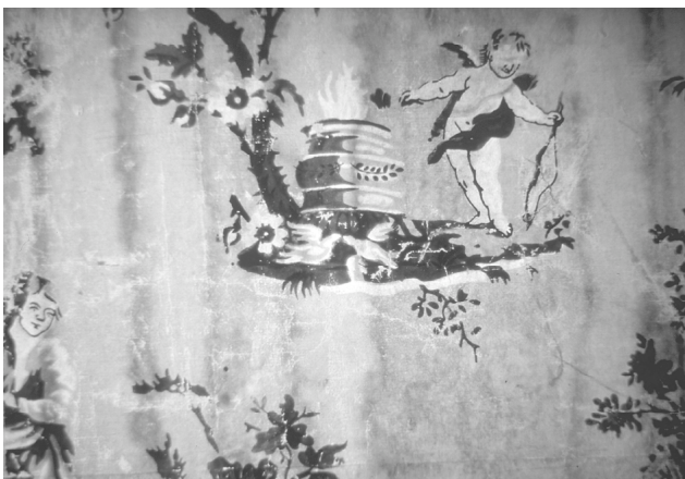
Fig. 14. Centreville stair hall, detail: after water emergency, before treatment
