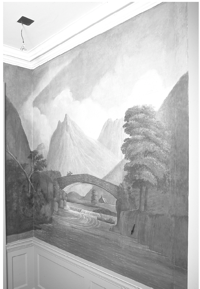
Fig. 3. Billiard room south alcove, after treatment
