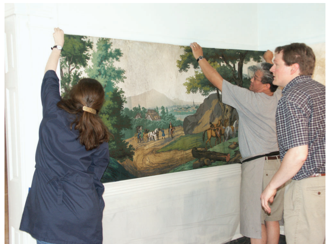
Fig. 17. Dianna Clise, Bryan Draper, and Michael Lee reinstall a section of wallpaper
