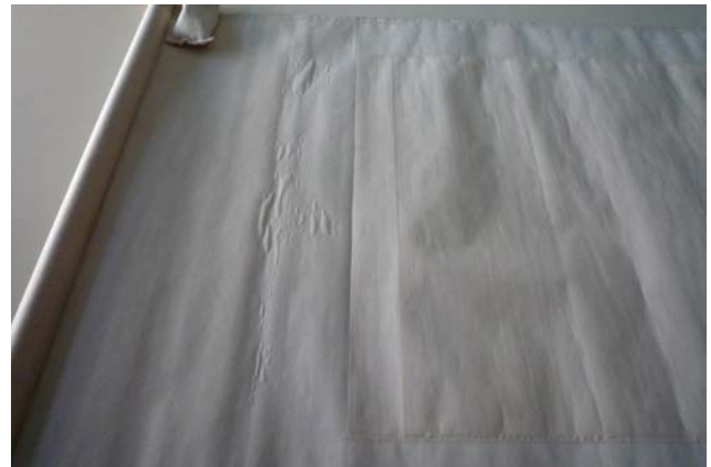
Fig. 12. Delamination between layers.
