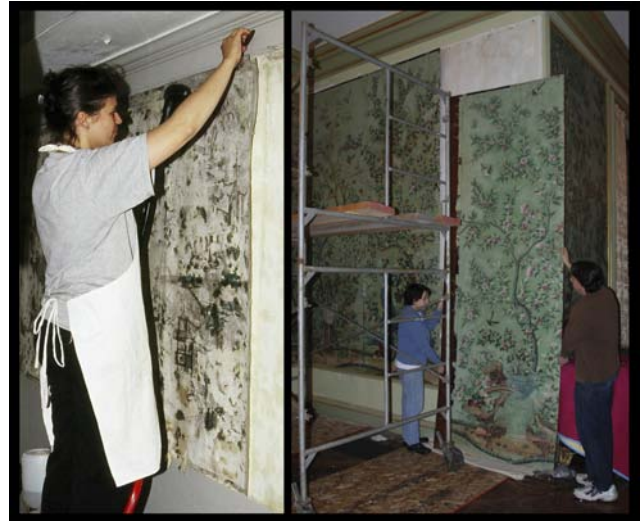
Fig. 4. Removal of Marblehead Chinoiserie and Newport Chinese export wallcoverings, photos Studio TKM.
