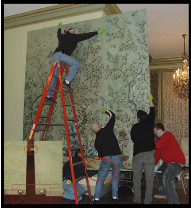
Fig. 10. Newport panels secured within moldings with detail of panel alignment hardware, photo Studio TKM.
